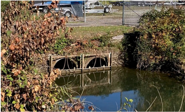
Stop plates at Marina Culvert
